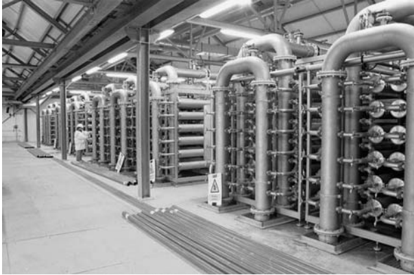
Fig. 7.5 Photograph of a 25-million gallon/day capillary hollow fiber module plant to produce potable water from a well, installed by Norit (X-Flow) in Keldgate, UK. Courtesy of Norit Membrane Technology B.
