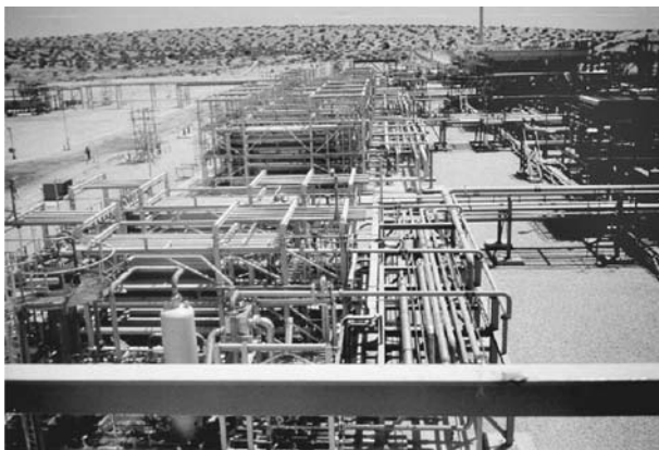
Fig. 7.11 A section of the Qadirpur, Pakistan, carbon dioxide removal plant built by UOP (Separex). The plant reduces the carbon dioxide content of natural gas from 6.5% to less than 2%. The original plant
