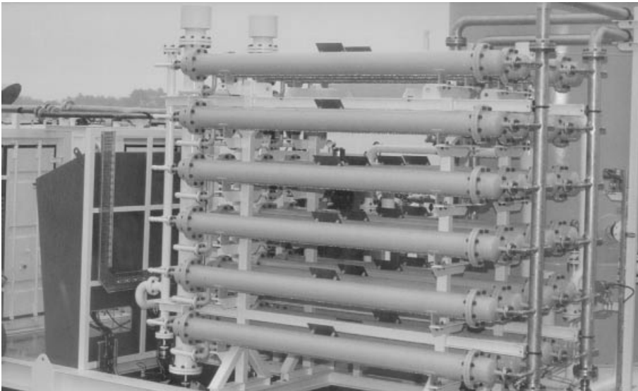
Fig. 2.7: Nitrogen generator for an off-shore platform. (Used with permission of Air Products and Chemicals, Inc.)
