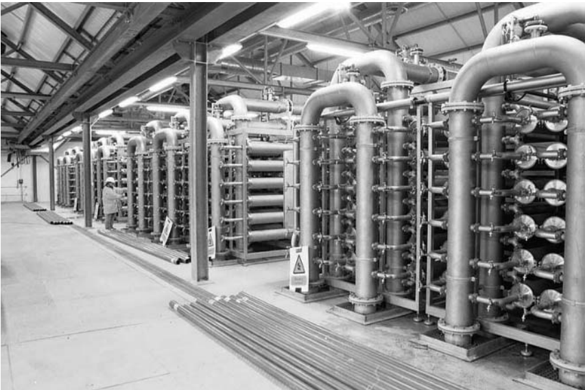
Figure 7.19 Photograph of a 25 million gal/day capillary hollow fiber module plant to produce potable water from a well, installed by Norit (X-Flow) in Keldgate, UK. Courtesy of Norit Membrane Technology BV
