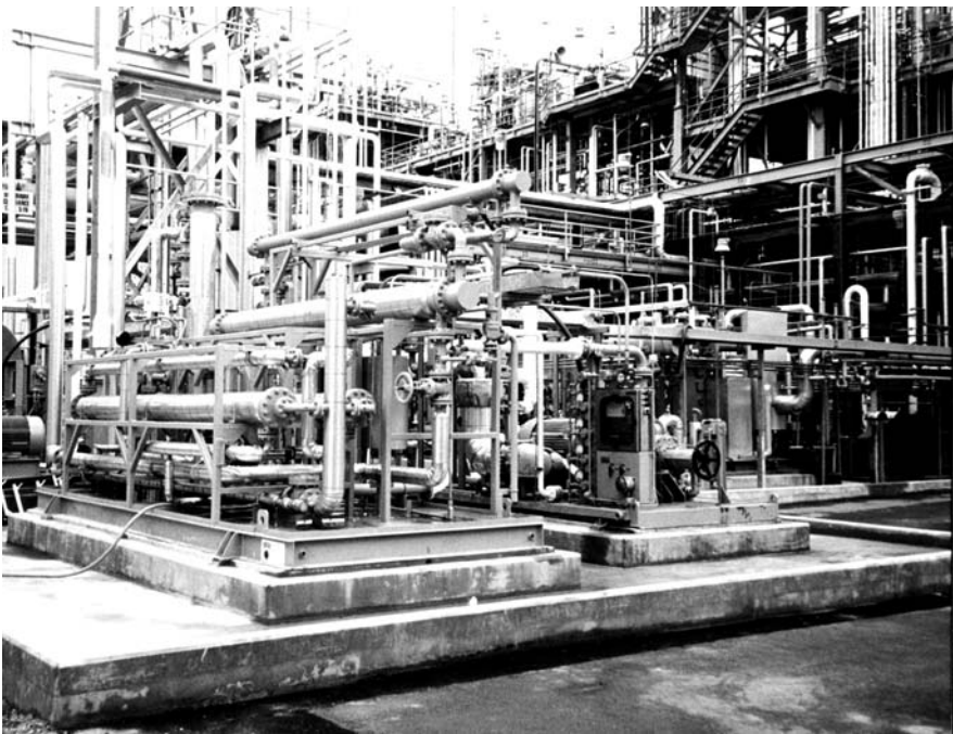
Figure 8.36 Photograph of a membrane unit used to recover nitrogen and propylene from a polypropylene plant vent gas
