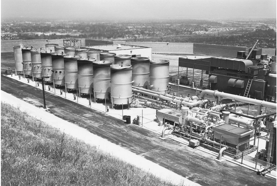
FIGURE 14.18 Large array of ground effects flares used to flare landfill gas.
