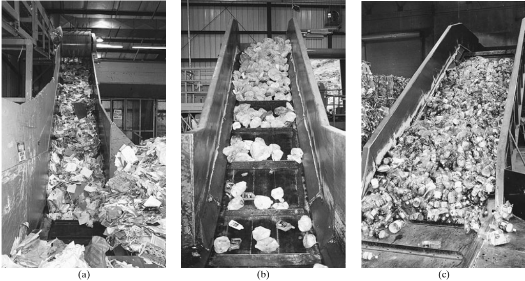
FIGURE 8.24 Inclined belt conveyors used to transport recyclable materials: (a) mixed paper to elevated sorting platform, (b) HDPE plastics to baler, and (c) PET plastics to baler.
