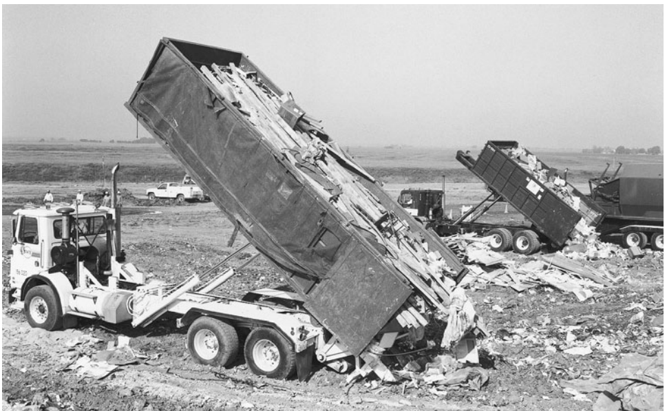
FIGURE 7.14 Contents of trash trailer used for demolition wastes being unloaded at landfill.
