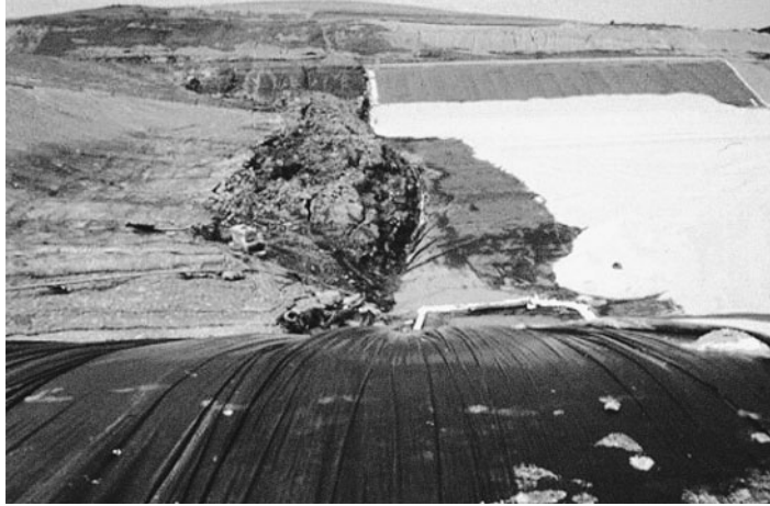
FIGURE 14.32 Landfill slope failure. ( Tim Stark, University of Illinois, 1998. )
