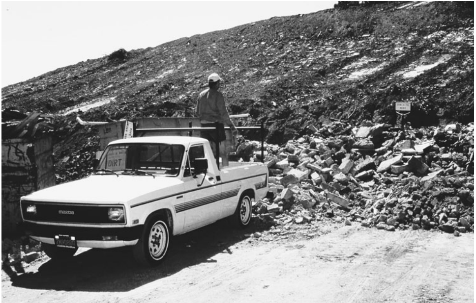
FIGURE 11D.1 Concrete demolition debris brought to a recycling center to be processed for reuse/recycling.
