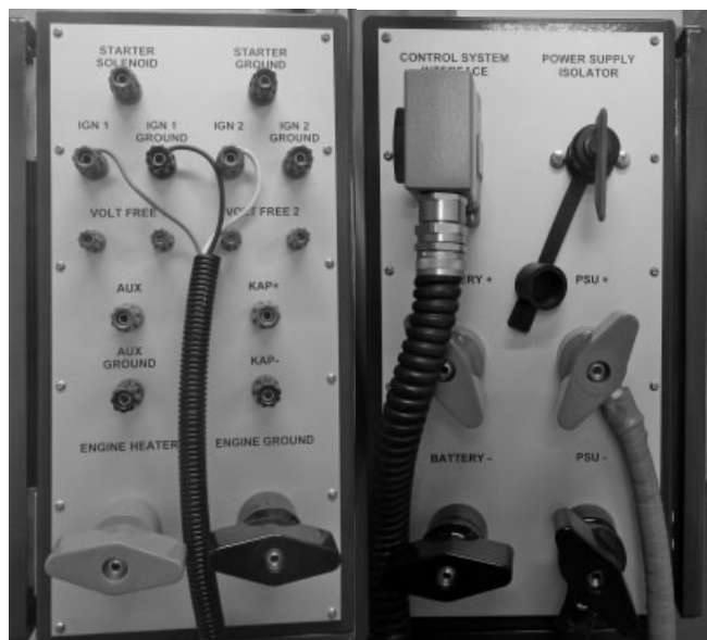
Figure 2. A composite photograph showing the two sides of an engine services box fitted within research cell testing both gasoline and diesel engines. (Photograph reproduced by permission of AVL-UK Ltd.)
