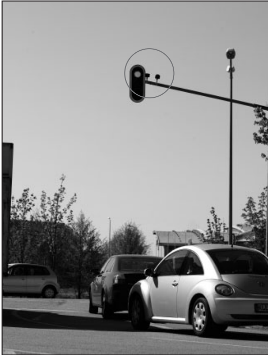
Figure 6. Typical installation of radar detectors.
