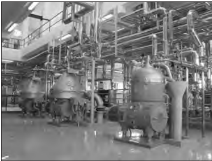
FIGURE 8–41 A piping network in an industrial facility.
