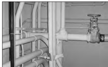
Piping and plumbing systems Photo by John M. Cimballa.
