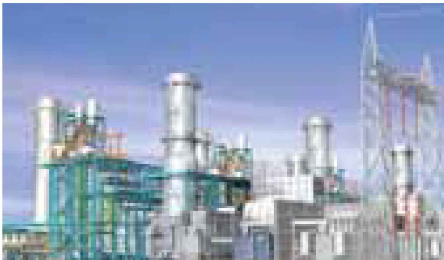
In power plants turbines and pipes function under high temperatures and pressures.
