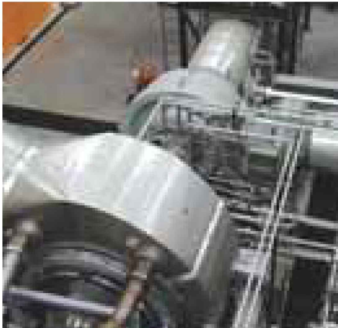
Gas turbine generator control system.
