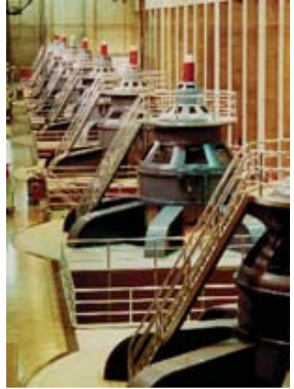
A series of hydel generators.
