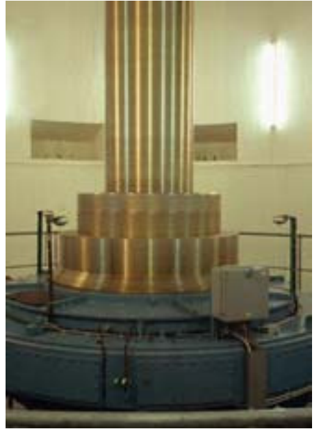
A big hydel generator. Governors are used to control the supply of working fluid (water in hydel generators).
