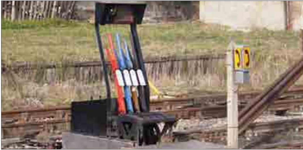
These levers are used to change railway tracks.
