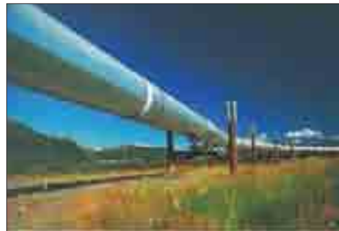
The Trans-Alaska Pipeline carries crude oil 1,284 kilometres through Alaska. The pipeline is 1.2 metres in diameter and can transport 318 million litres of crude oil a day.
