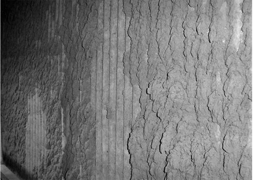
Figure 24: Example of fouled water tube furnace wall [23].
