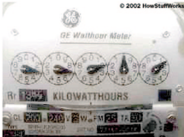
Fig. 17.16 Typical power meter. (Courtesy of PG&E)
