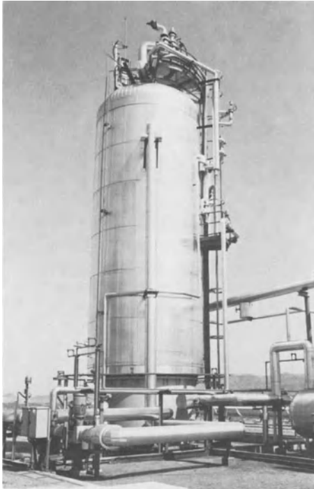
Fig. 58. View of storage tank, buffer tanks and hot oil pumps
