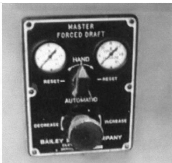
Figure 10-11. Early pneumatic H/A station
