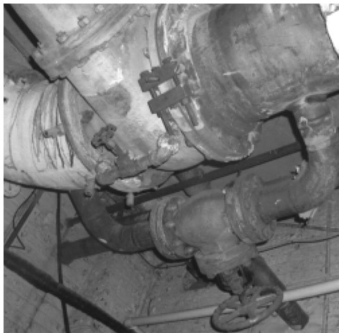
Figure 2-1. Warm-up bypass valves
