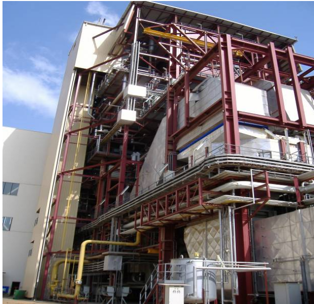
Figure 3. Example of a boiler of a TPP.
