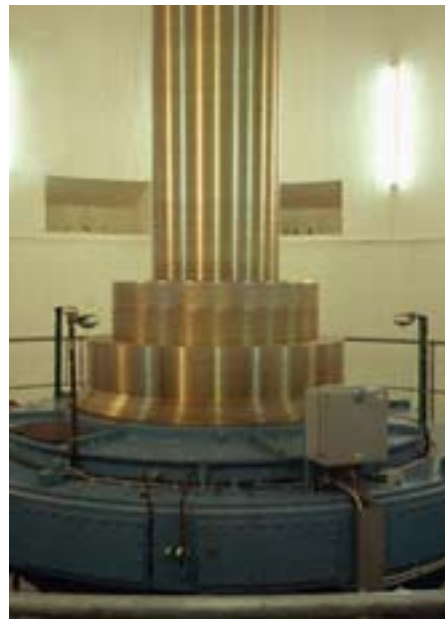
A big hydrel generator. Governors are used to control the supply of working fluid (water in hydrel generators).
