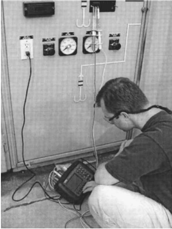
Figure 11.11 Demonstrating the use of a hand-held, three-phase power quality monitoring instrument to quickly evaluate voltages at the mains.
