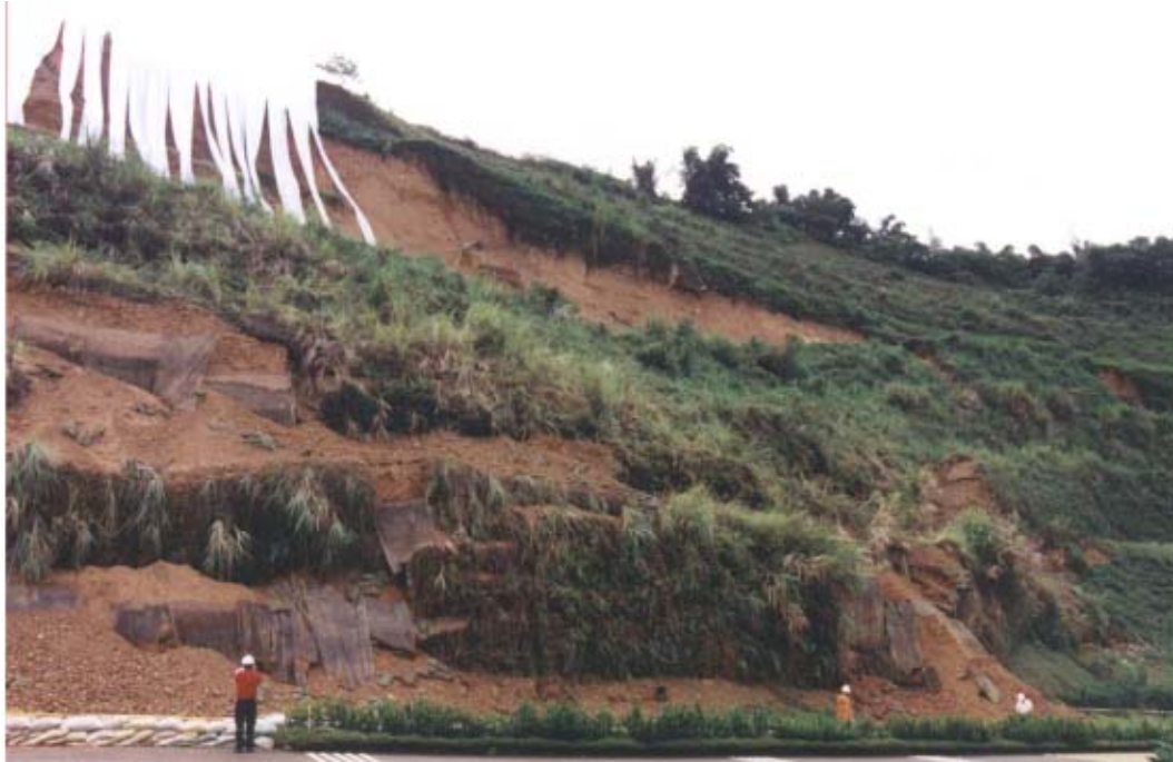
FIGURE 30.15 Fabric retaining wall damaged during the 1999 Ji Ji, Taiwan earthquake.
