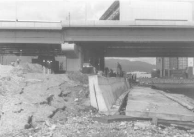
FIGURE 30.7 Liquefaction-caused bridge damage during Kobe earthquake.
