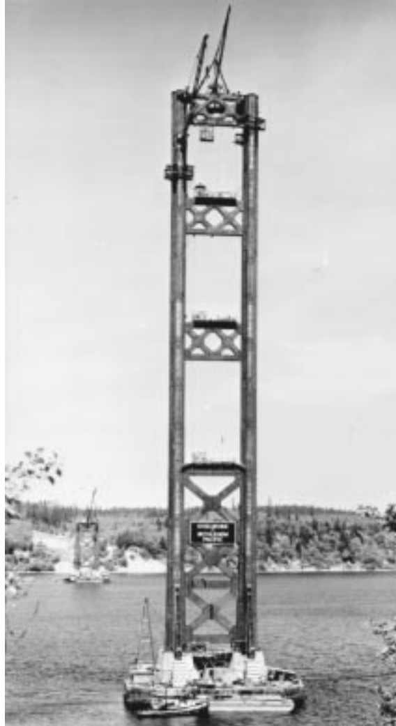
FIGURE 20.24: Tower erection, second Tacoma Narrows Bridge, Washington, 1949. This bridge replaced first Tacoma Narrows bridge, which blew down in a 40-mph (18-m/sec) wind in 1940. The tower legs are 60 ft (18 m) on centers and 462 ft (141 m) high. The creeper traveler is shown erecting the west tower, in background. On the east tower, the creeper erected a Chicago boom at the top of the south leg; this boom dismantled the creeper, then erected the tower-top bracing and a stiffleg derrick, which proceeded to dismantle the Chicago boom. The tower manhoist can be seen at the second-from-topmost landing platform. Riveting cages are approaching the top of the tower. Note tower-base erection kneebraces, required to ensure tower stability in free-standing condition (see Figure 20.27).
