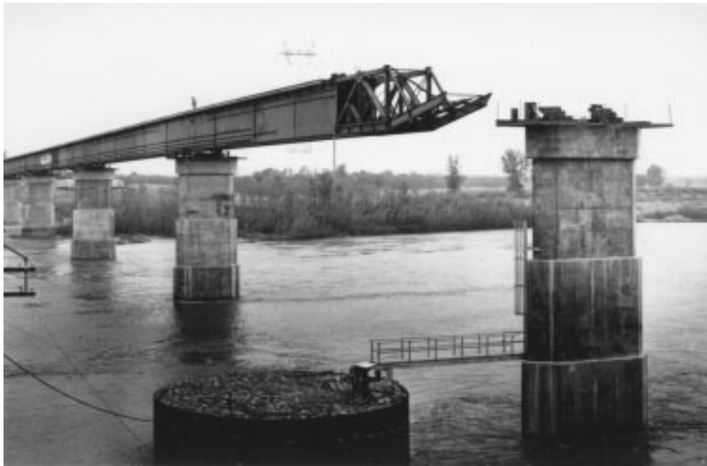
Figure 20.41a Leading end of north girder train moves across 250-ft (76-m) span 4, approaching pier 5. Main span is to right of pier 5.
