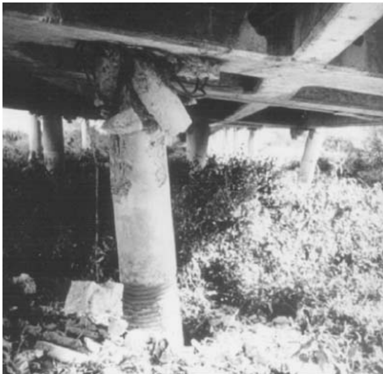
FIGURE 30.25 Broken piles under the bridge.
