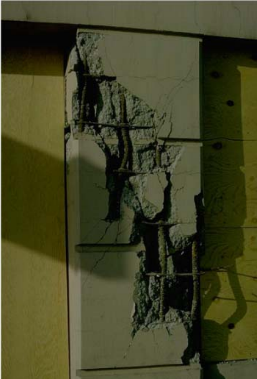
FIGURE 30.50 Damage to the south side of Mt. McKinley Apartments. (Photograph by Karl Steinbrugge and courtesy of the Steinbrugge Collection, Earthquake Engineering Research Center, University of California, Berkeley.)
