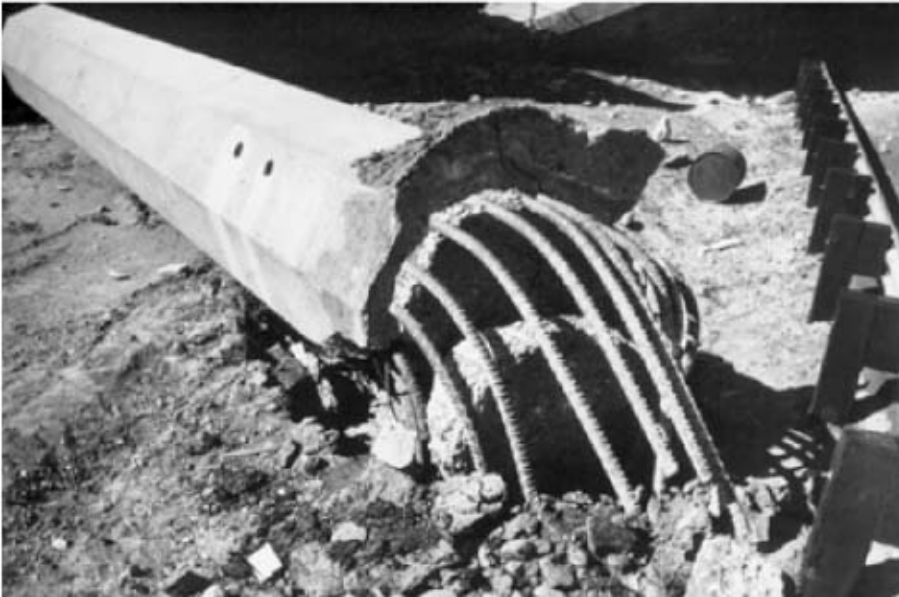
FIGURE 30.35 Failure of connection of column to pile shaft.
