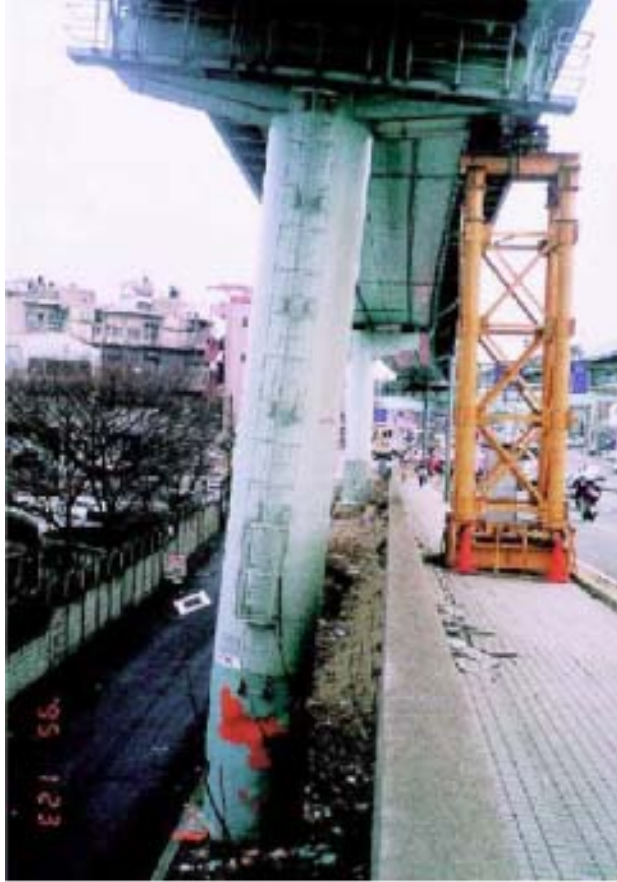
FIGURE 30.54 Pier 585 on Kobe Route 3 during the 1995 Kobe earthquake. (Courtesy of Hanshin Expressway Public Corporation.)
