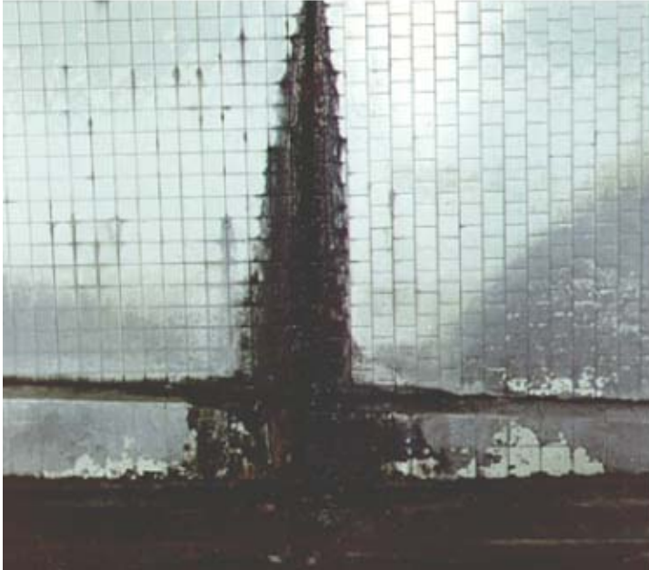
FIGURE 30.10 Liquefaction-induced damage to Webster Street Tube tunnel.
