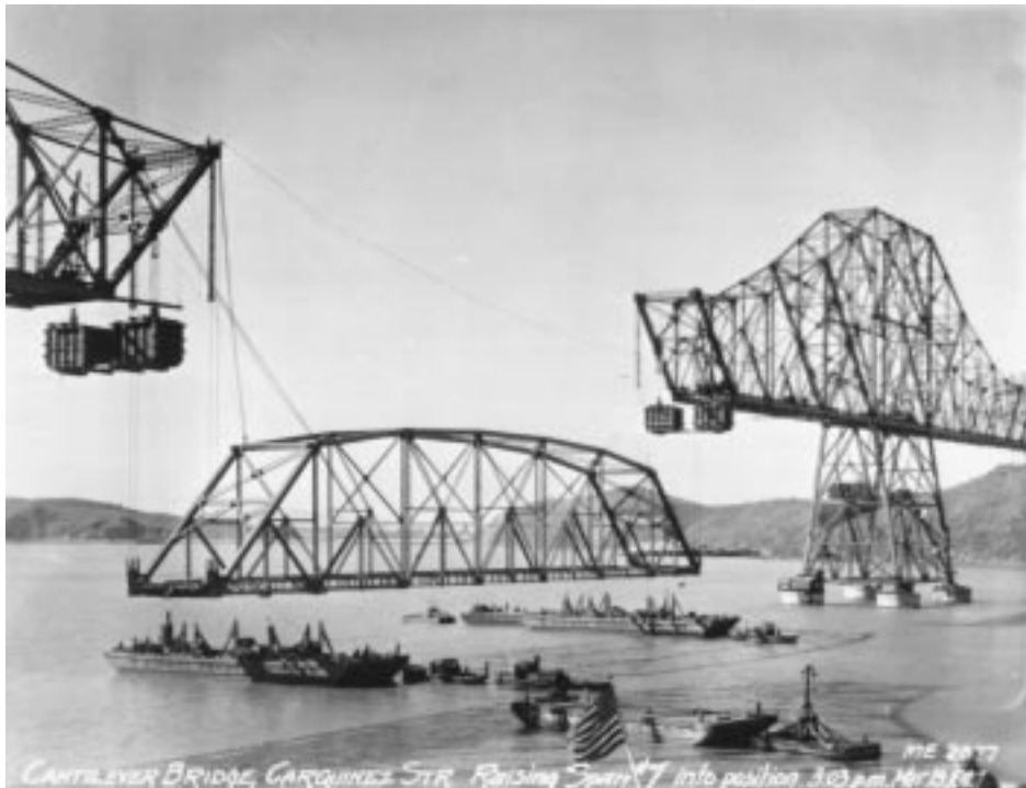
FIGURE 20.20: Raising of suspended span, Carquinez Strait Bridge, California, 1927. The 433-ft (132-m) suspended span, weighing 650 tons, was raised into position in 35 min., driven by four counterweight boxes having a total weight of 740 tons.
