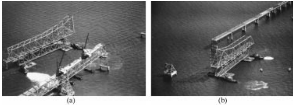
FIGURE 20.30: Floating-in erection of a truss span, first Chesapeake Bay Bridge, Maryland, 1951. Erected 300-ft (91-m) deck-truss spans form erection dock, providing a work platform for two derrick travelers. A permanent deck-truss span serves as a falsework truss supported on barges and is shown carrying the 470-ft (143-m) anchor arm of the through-cantilever truss. This span is floated to its permanent position, then landed onto its piers by ballasting the barges. (a) Float leaves erection dock, and (b) float arrives at permanent position. (Courtesy of Bethlehem Steel Corporation.)
