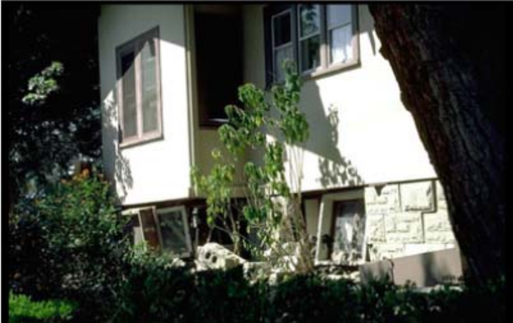
FIGURE 30.32 Hollow concrete-block foundation that failed during the magnitude 6.0 1987 Whittier, CA earthquake. (Photograph by Karl Steinbrugge and courtesy of the Steinbrugge Collection, Earthquake Engineering Research Center, University of California, Berkeley.)
