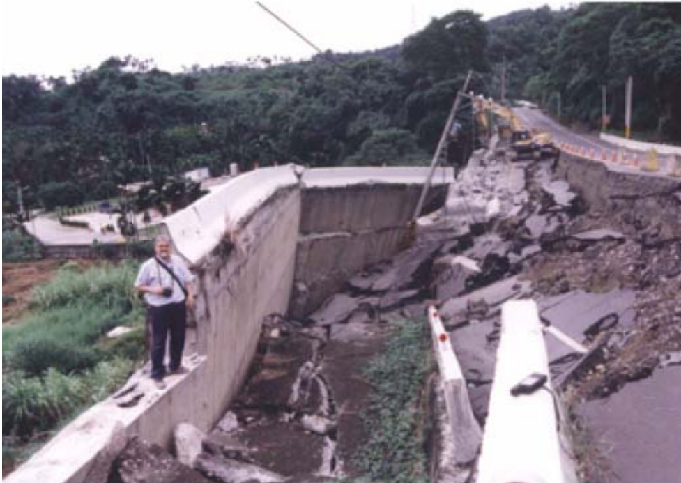
FIGURE 30.13 Gravity retaining wall pushed outward by landslide.
