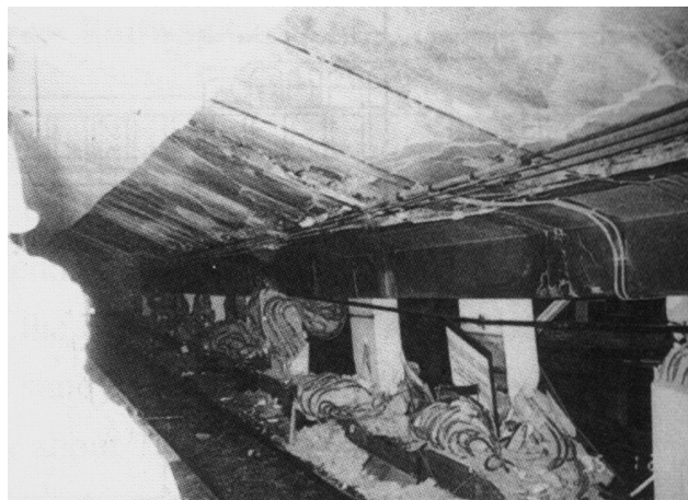
FIGURE 30.53 Flexural damage to columns at lower-level of Dakkai Subway during the 1995 Kobe earthquake. (Courtesy of Japan Society of Civil Engineers [5].)
