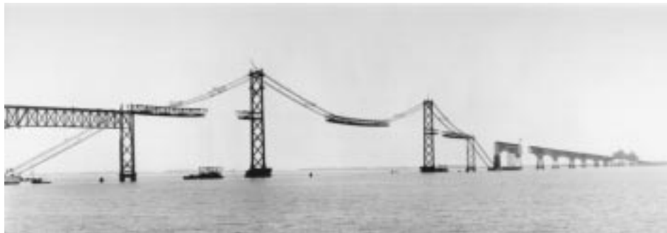
FIGURE 20.6: Suspension spans of first Chesapeake Bay Bridge, Maryland, 1952. Deck steelwork is under erection and is about 50% complete. A typical four-panel through-truss deck section, weighing about 100 tons, is being picked in west side span, and also in east side span in distance. Main span is 1600 ft (488 m) and side spans are 661 ft (201 m); towers are 324 ft (99 m) high. Cables are 14 in. (356 mm) in diameter and are made up of 61 helical bridge strands each (see Figure 20.8).
