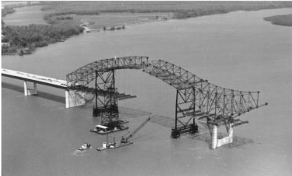
FIGURE 20.43: Erection of west arch span of twin-arch Hernando de Soto Bridge, Memphis, Tenn., 1972. The two 900-ft (274-m) continuous-truss tied-arch spans were erected by a high-tower derrick boat incorporating a pair of barges. West-arch steelwork (shown) was cantilevered to midspan over two pile-supported falsework bents. Projecting east-arch steelwork (at right) was then cantilevered to midspan (without falsework) and closed with falsework-supported other half-arch. (Courtesy of Bethlehem Steel Corporation.)
