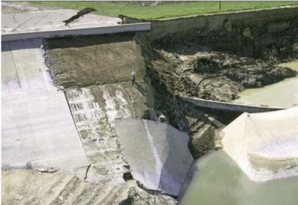
FIGURE 30.22 Closer view of damage to the Lower San Fernando Dam. (Courtesy of Steinbrugge Collection, Earthquake Engineering Research Center, University of California, Berkeley.)
