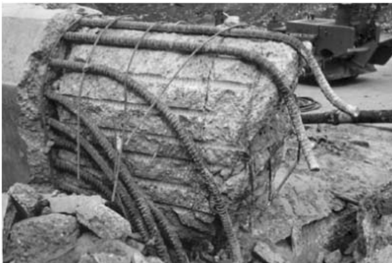
FIGURE 30.36 Failure of connection of column to footing.
