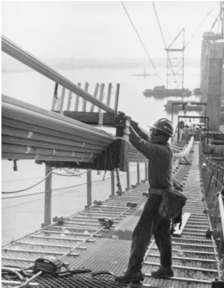
Figure 20.37b Cable formers maintain strand alignment in cables prior to compaction. Each finished cable is about 15-1/4 in. (387 mm) in diameter. (Courtesy of Bethlehem Steel Corporation.)
