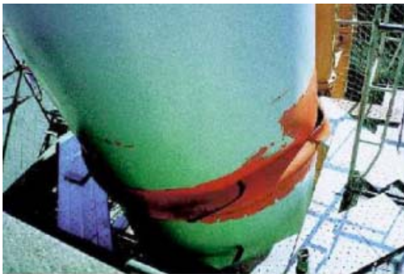
FIGURE 30.55 Torn buckle of steel column on Route 3 after the 1995 Kobe earthquake. (Courtesy of Hanshin Expressway Public Corporation.)
