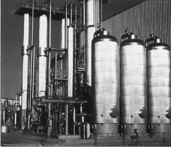
Fig. 5a. Pressure swing adsorption beds for the dehydration of alcohols ( courtesy of Howe-Baker Engineers )
