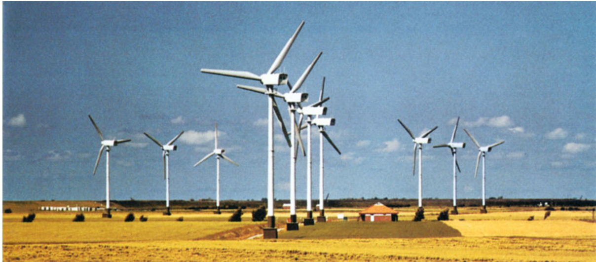
Figure 8.49 Windfarm Krummhörn. Rotor span width is 30 m, the nominal electric power output is 300 kW per wind converter. (With kind permission of EWE corporation, Oldenbourg)
